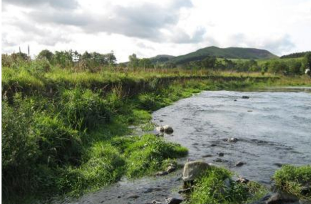
Before - the eroded riverbank at Clifton-on-Bowmont
